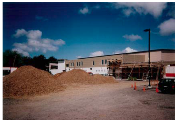
Using crushed concrete as aggregate is an easy way to specify recycled products.
