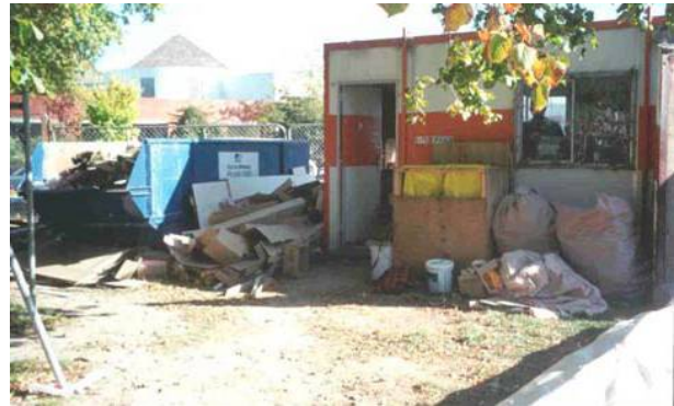
Sorting waste, Hawkins Construction, Christchurch. From left to right: Timber pile, blue landfill skip, cardboard pile for recycling, yellow hazardous waste bags (landfill), soft plastic for recycling.
