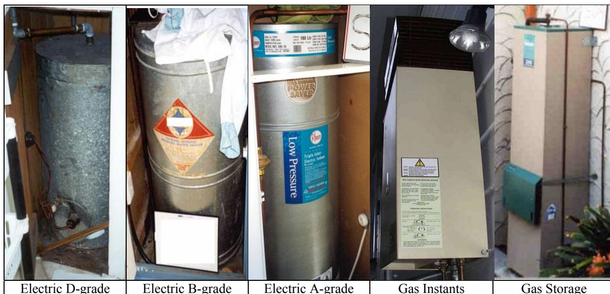
Figure 52: Examples of hot water cylinders
